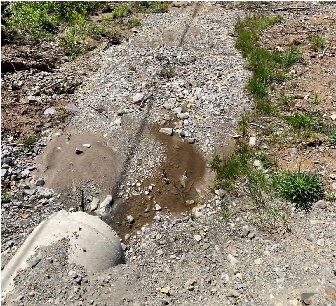
Figure 5. Photograph taken on 24 May 2022 showing the concrete culvert installed within the ditch adjacent to Base Road for accessing 28 Base Road in Garnett Settlement, New Brunswick.
