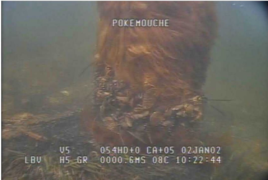
T7: Soft sour weed on wooden column in the 20-25m segment.
