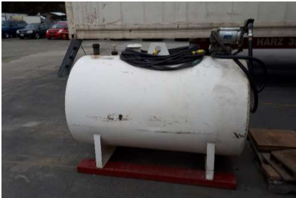
Photo No. 14: View of 1120-L Portable Aboveground Fuel Oil Tank Located by Effluent Filtration Building
