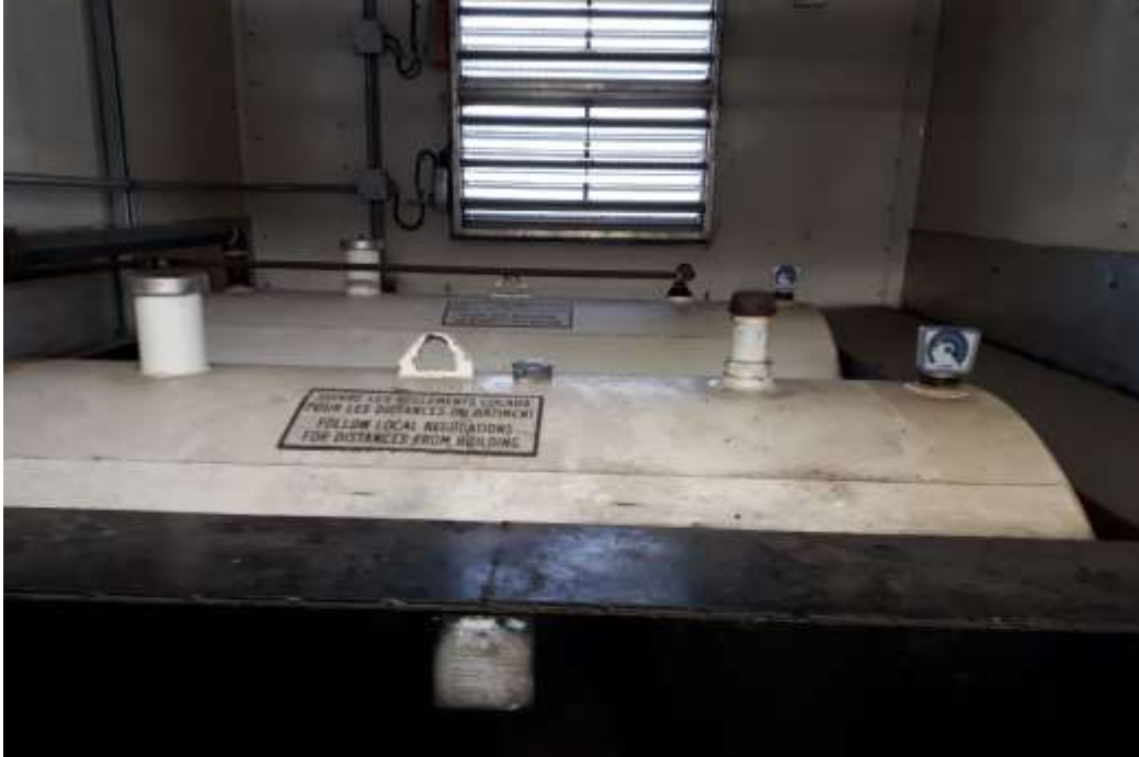
Photo No. 13: View of Two Aboveground Fuel Oil Tanks (2250 L Capacity Each) Located Inside Portable Boiler Unit
