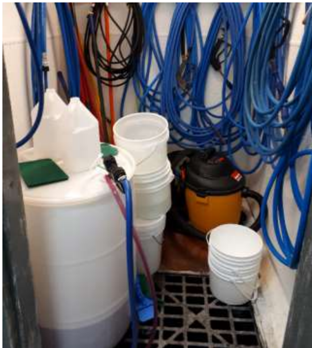
Photo No. 20: View of Chemical Storage (with secondary containment) Inside the Plant
