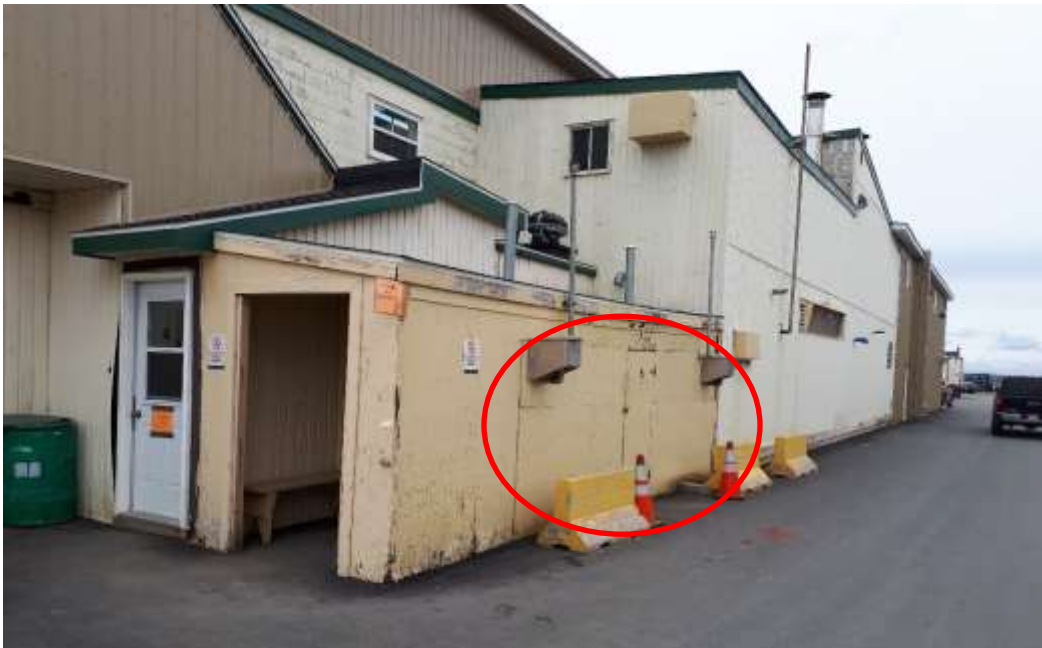
Photo No. 10: Location of Two (2) 2380L Aboveground Fuel Oil Tanks (Circled in Red)
