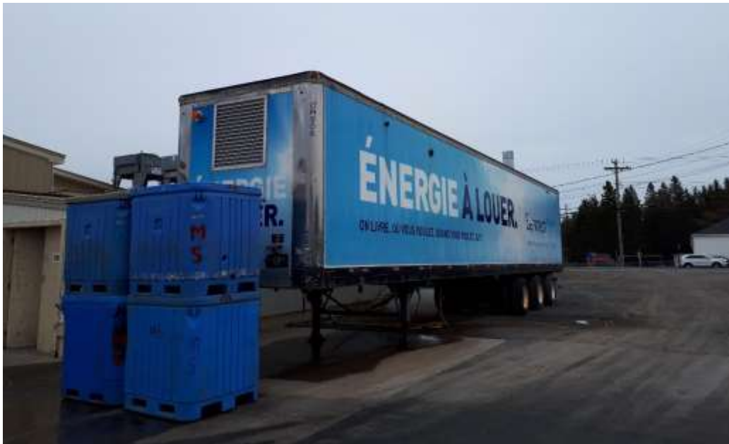
Photo No. 12: Portable Crab Boiler Unit (Exterior)
