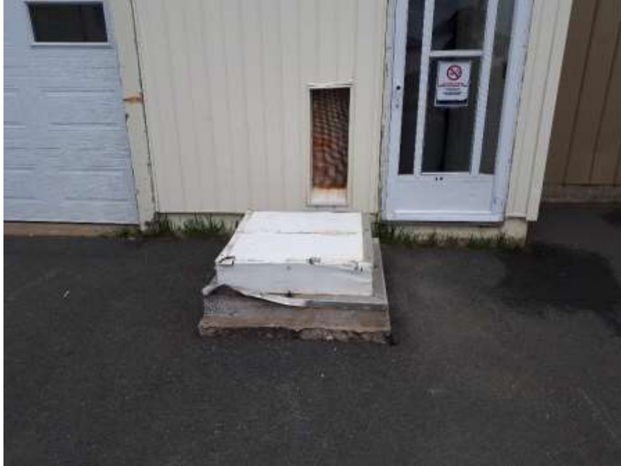
Photo No. 1: Production Well No. 1 (PW1)
