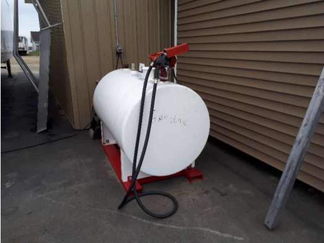
Photo No. 15: View of 1120-L Portable Aboveground Gasoline Tank Located in Outside Yard
