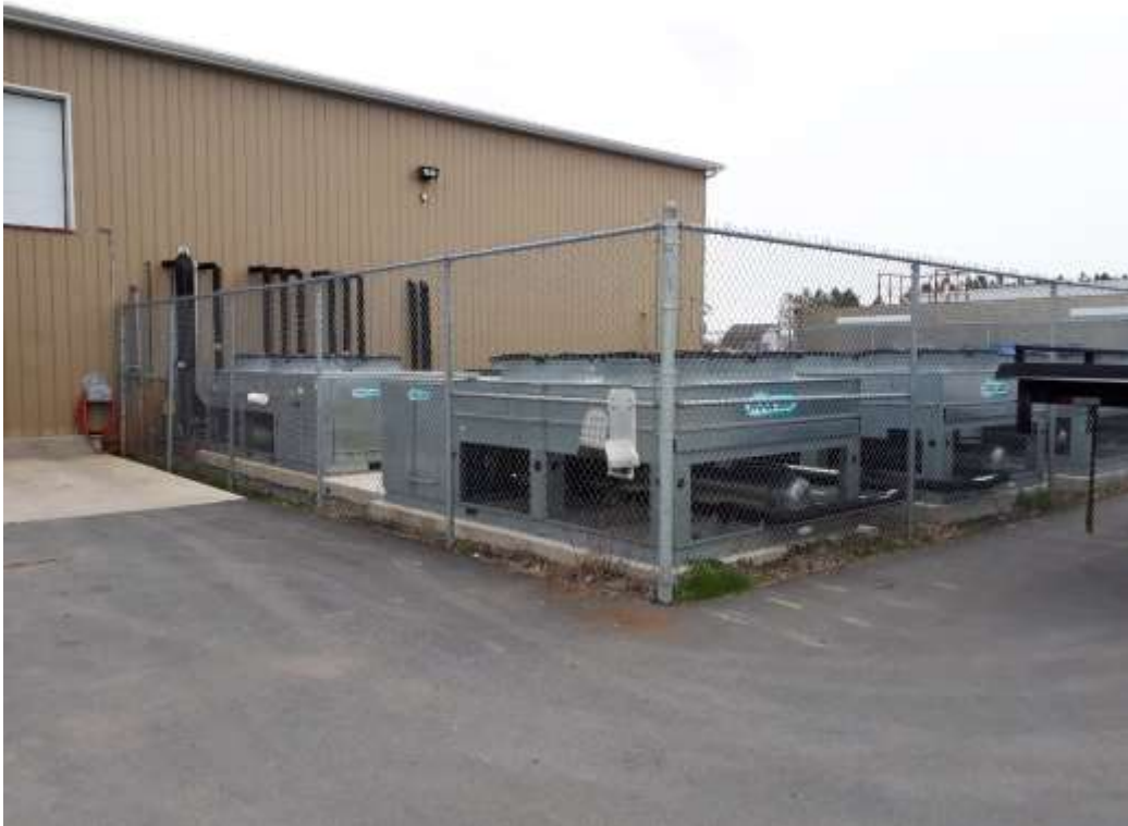
Photo No. 16: Refrigeration Compressors
