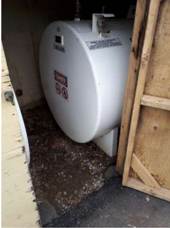
Photo No. 11: View of One of the 2380-L Aboveground Fuel Oil Tanks
