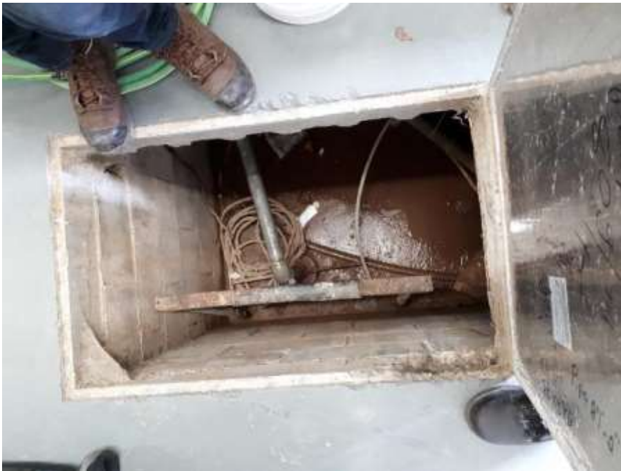
Photo No. 2: Production Well No. 2 (PW2)
