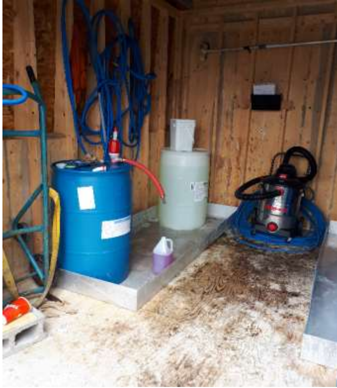
Photo No. 19: View of Chemical Storage (with secondary containment) Inside of Storage Shed
