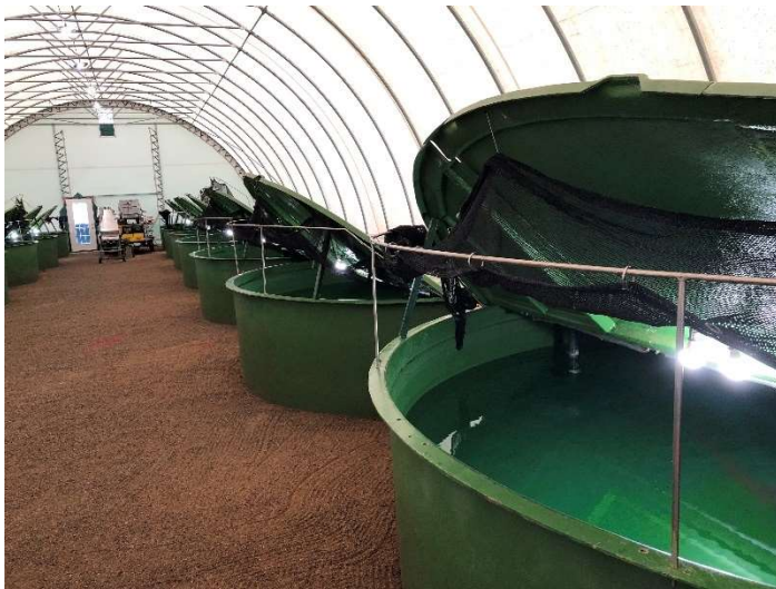
Figure 6 Existing First Feed Tanks
