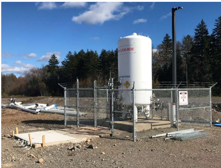
Figure 8 Liquid Oxygen Storage Tank
