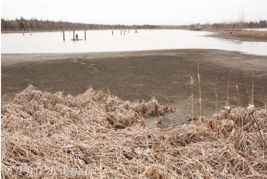
Figure 7-3a Vegetation Growing on Area of Exposed Sediment Along the Top of Cell No.2 of the ASB Looking Towards the Electrical Building on Left (Same area as Figure 7-3b but taken May 2014)
