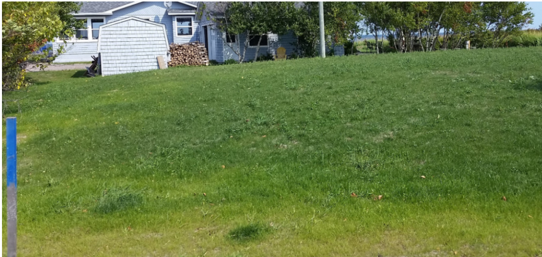
Mound system in Area 2
