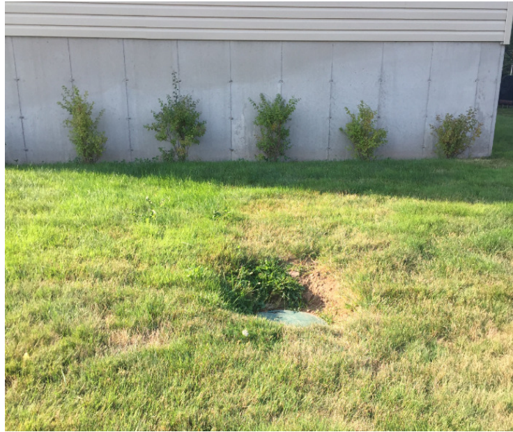
Holding tank in Area 1A
